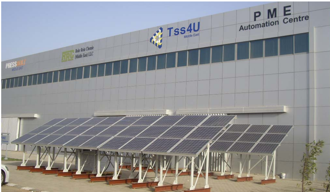
The 1200Wc system in front of the Tss4U Middle East facility.
